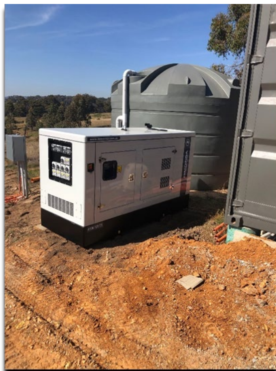
Temporary generator to power the site
